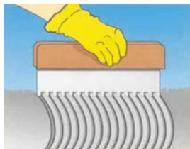
Spreading of Sikafloor®-262 AS N with notched trowel. E.g. Polyplan notched trowel 5/7 mm.
